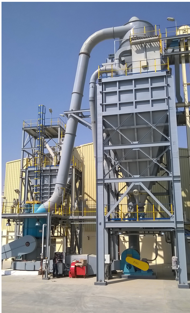
Figure 1. Bradley airswept mill system.
